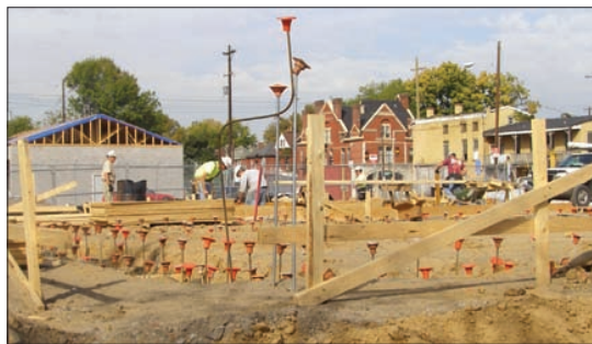
Workers at a construction site along the St. Catherine Street curve between Jackson and Preston streets are working on part of the expansion of the Society of St. Vincent de Paul campus. The $10.6 million project will transform an entire city block.
